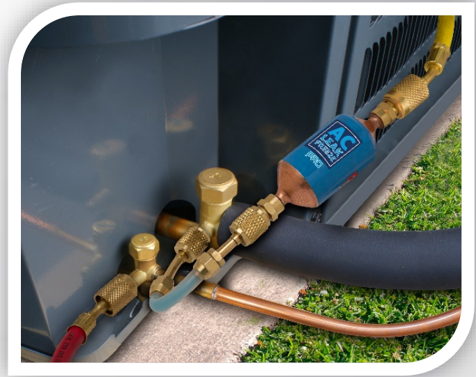
AC Leak Freeze
