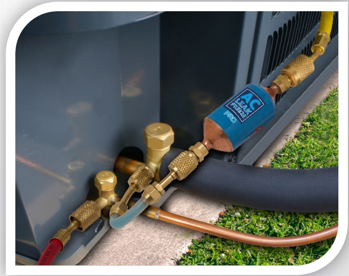
AC Leak Freeze
